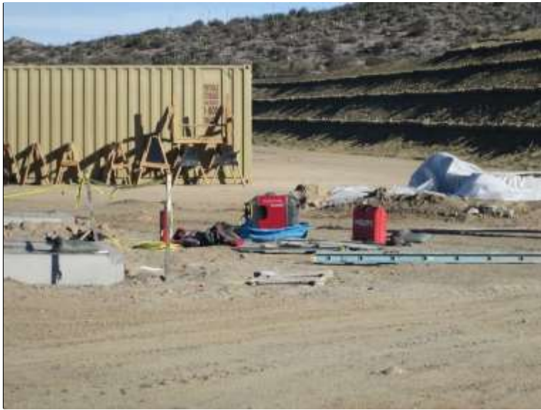
Photo 7: Staged equipment and portable facilities equipped with containment measures in accordance with HAZ-1a.
