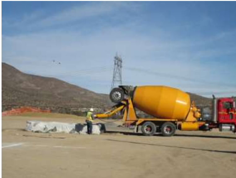
Photo 8: A concrete washout bin was observed being utilized and maintained in good condition in accordance with the SWPPP and MM-HYD-1.
