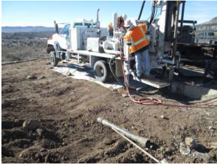
Photo 5: Stationary equipment placed on plastic sheets to prevent potential leaks from being discharged into the soil as per MM HYD-1.
