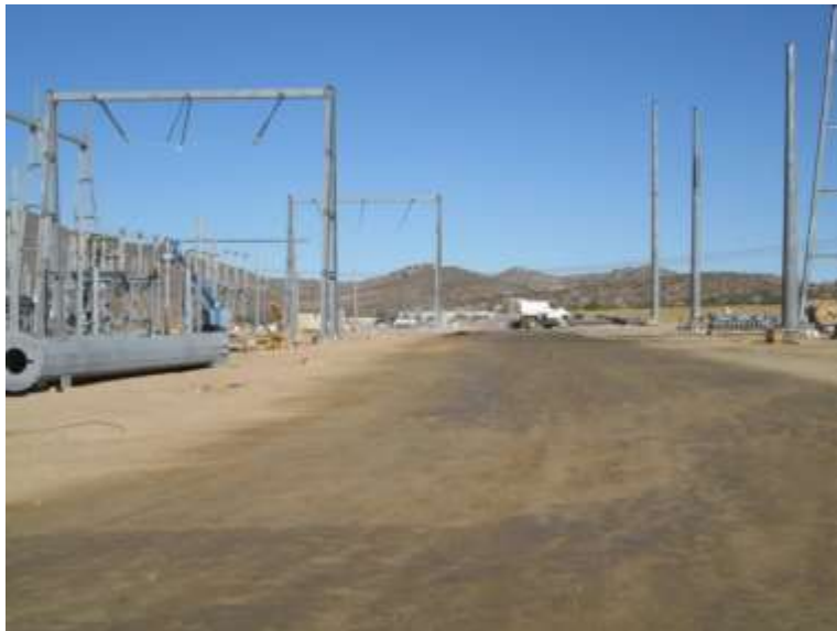
Photo 6: Water trucks applying water to areas of active construction on a regular basis to minimize fugitive dust emissions.
